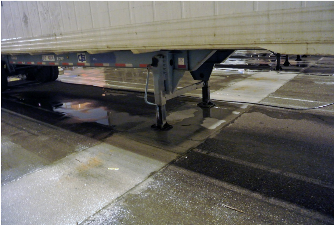
Figure 5. Concrete apron installed to support container chassis landing gear
